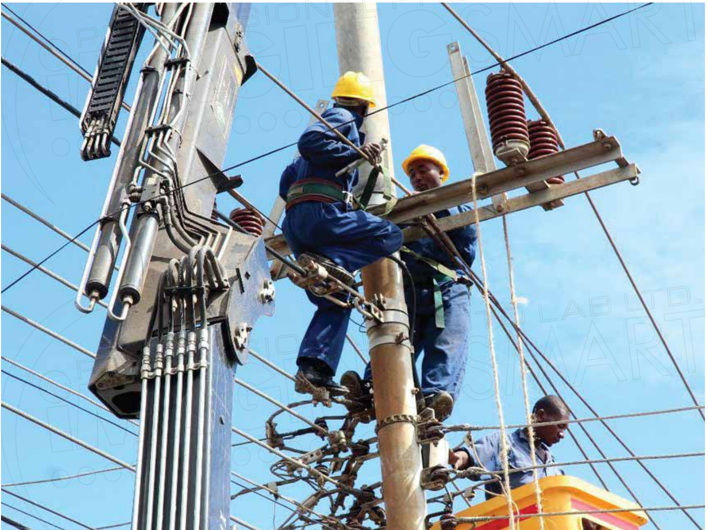
Workers on a power transmission line: Discipline is the mother of safety; safety begets productivity and zero compensation claims thereby enhancing financial wellbeing. Photo: https://www.powertelcom.com/tanzania-project/
