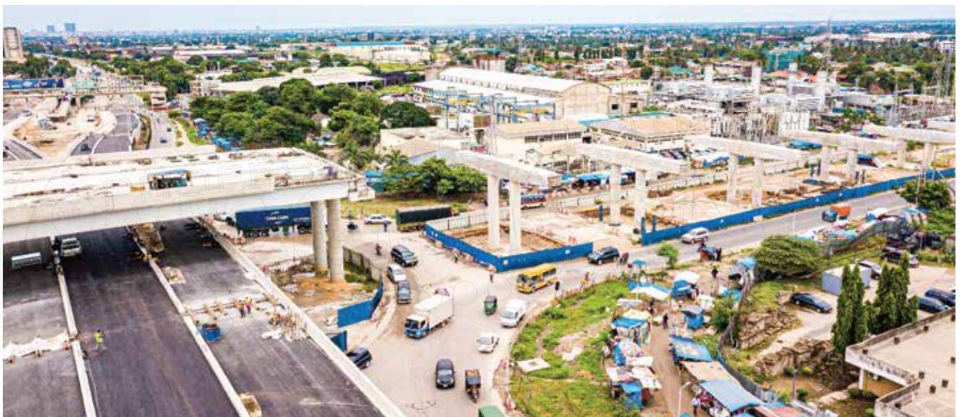
Discipline means willingness to safely share limited space with others and following schedules to avoid costly accidents, for example: Ubungo interchange construction project site, Dar es Salaam. [Photo: Tanroads website]
