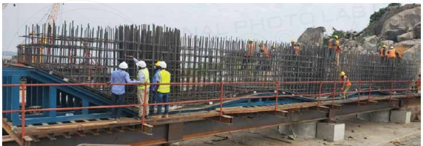
Discipline engenders respect and harmonious working relationship at construction site, boosting productivity and minimizing accidents and compensation claims: Workers at Magufuli Bridge Project, Mwanza: [Photo: Tanroads website]
