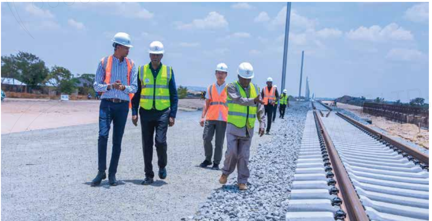
Every construction activity carries a financial weight which can be made light by a carefully drawn project plan and budget: Some Members of Contractors Registration Board, its Chairman Eng. Joseph Nyambanga (Front, right), its Registrar Eng. Rhoben Nkori and members of its management, inspect construction of 341kilometre SGR line from Mwanza to Isaka, in the company of contractors, at Malampaka, Shinyanga, recently.
